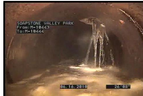
Extensive Water Infiltration
