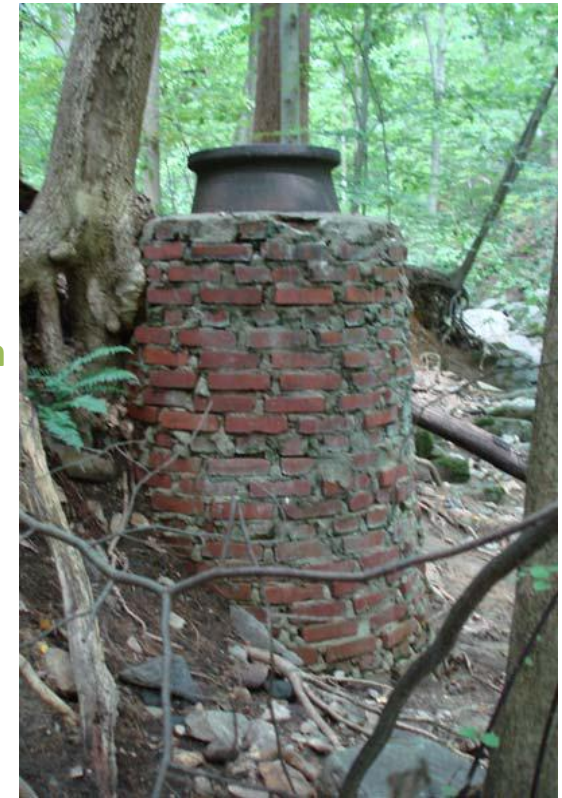
Manhole Exposed by Erosive Stream Channel
